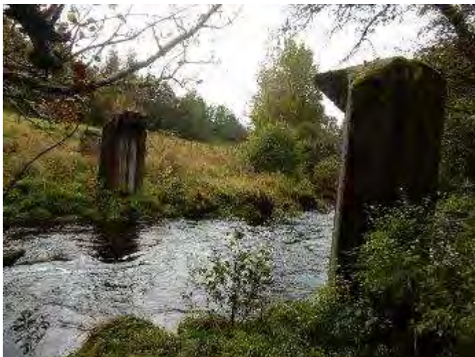
Stanchions of former bridge across the River Deveron still in place but would require structural survey to assess scope to rebuild build, cost and implications
