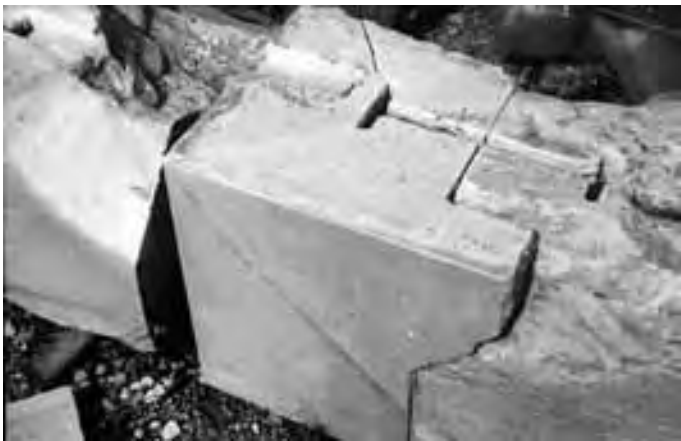
Figure 133. The Erechtheion: a block of marble restored by Balanos. The original stone has been cut in order to accommodate new marble. Iron cramps have since caused cracking of the original stone
