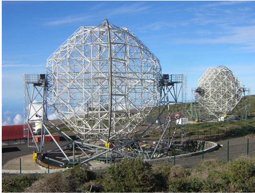
The two MAGIC telescopes in November 2006. The nearest instrument is MAGIC-II and is currently undergoing installation of its main components.
