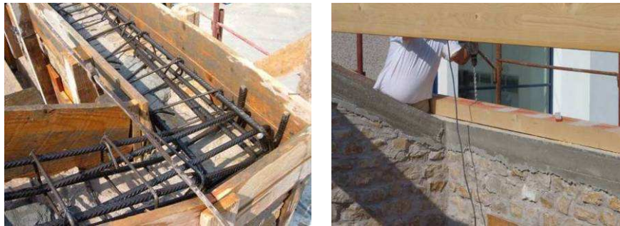
Figure 2. Detail of the reinforcement of the joint at the base of the gable wall (left). Operation of drilling the timber spreader beam and the concrete ring beam (right)
