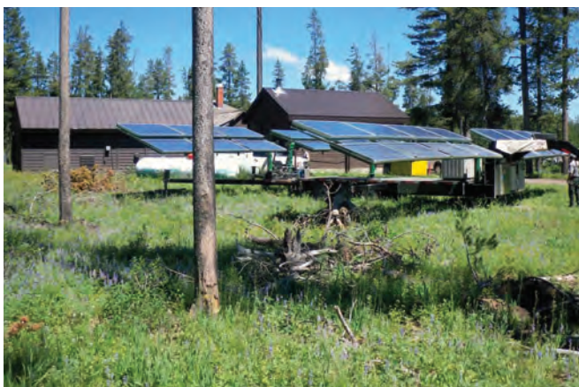
This portable photovoltaic system at Bechler provides power during the summer season, meeting 90% of the site's electrical needs.
