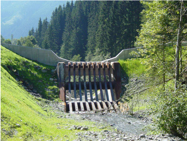
Fig. 2 View of a large slot grill barrier for dosing and filtering
