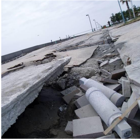
(c) Road at unimproved area after earthquake.
