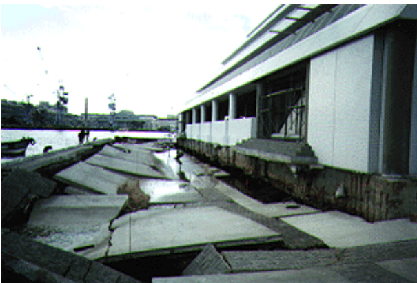
(a) Damage of sea revetment near the building.
