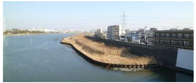
(b) River embankment after earthquake.
