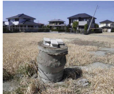
Figure 16. Floating of sewage manhole (Itako, Ibaragi).
