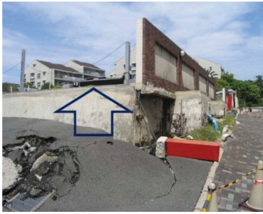
Figure 15. Floating of underground parking structure (Yokohama).
