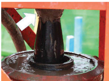
Figure 62. Plastic drain caught by rotation of jet grouting machine.
