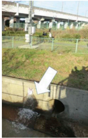
Figure 55. Discharge of ground water into river in Kuki City (photo provided by Prof. J. Koseki).
