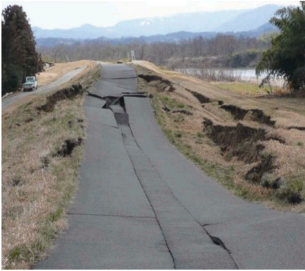
Figure 20. Crest subsidence and lateral spreading of Abukuma-River levee (Sasaki et al., 2012).
