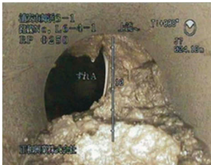
Figure 70. Flow-in of liquefied backfill sand into separated sewage pipes (photograph by Urayasu City).
