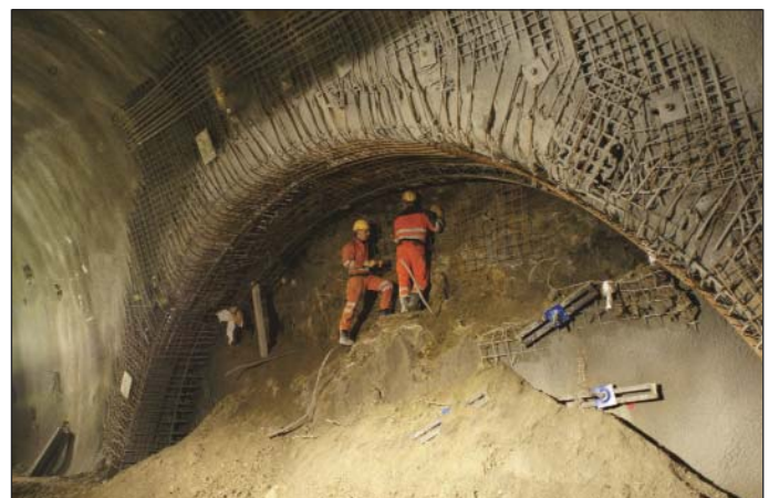
Obr. 6 Vystužovanie prieniku severnej tunelovej rúry s prístupovou štôľňou Fig. 6 Installation of concrete reinforcement at the intersection between the northern tunnel tube and the access tunnel
