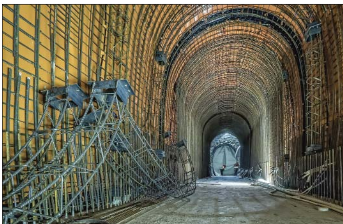
Obr. 3 Kolektorová trasa J102–TK103 – montáž armatury kleneb Fig. 3 Utility tunnel route J102–TK103 – installation of reinforcement of vaults
