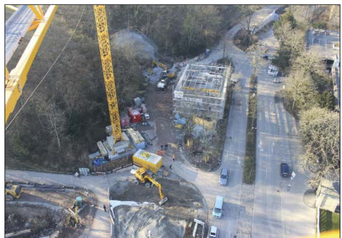
Obr. 3 Celková stiesnená plocha zariadenia staveniska s portálom prístupovej štôlne na bývalom autobusovom parkovisku ZOO Wilhelma Fig. 3 The overall confined area of the construction site facilities with the portal of the access tunnel on the former ZOO Wilhelma bus parking lot
