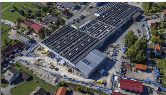
Obr. 11 Zastavané územie Gießenbach nad tunelom (Firma Langmatz – injektážne šachty a odvodňovacie potrubie) Fig. 11 Developed Gießenbach area above the tunnel (Langmatz company – shafts for injecting grout and a drainage pipeline)
