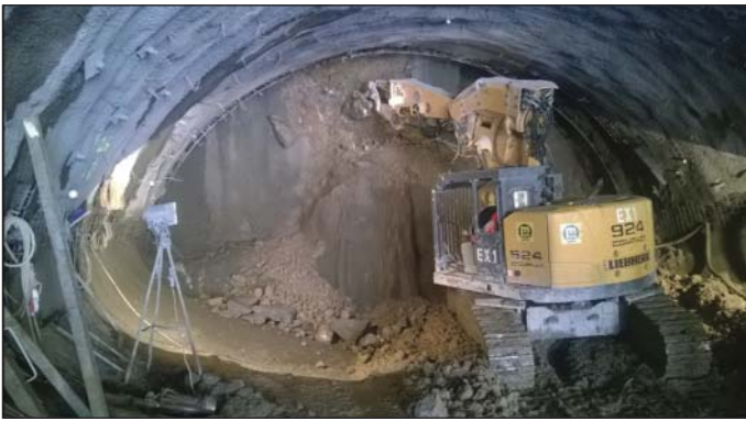
Obr. 6 Raziace práce v oblasti Gießenbach (delené otváranie čelby) Fig. 6 Tunnel excavation operations in the Gießenbach area (sequential excavation)
