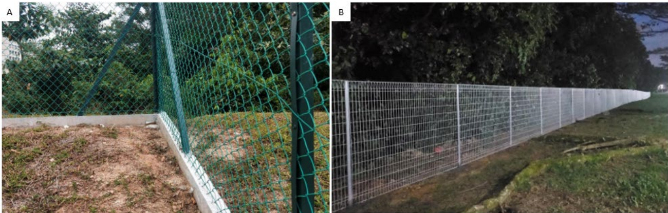
Figure 55: (A) Fences with cement base to prevent animals from burrowing through them; (B) BRC or weldfences along a vegetated area at Pasir Ris Park
