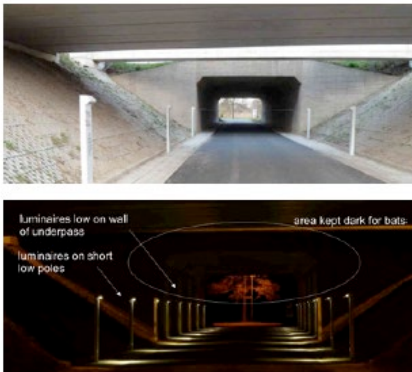
Figure 50: Installation of luminaires on short poles to reduce artificial light at night on a commuting route for bats through an underpass in the Netherlands (the same place in daylight and at night). Source: Voigt et al. (2018); photograph by F. Brekelmans
