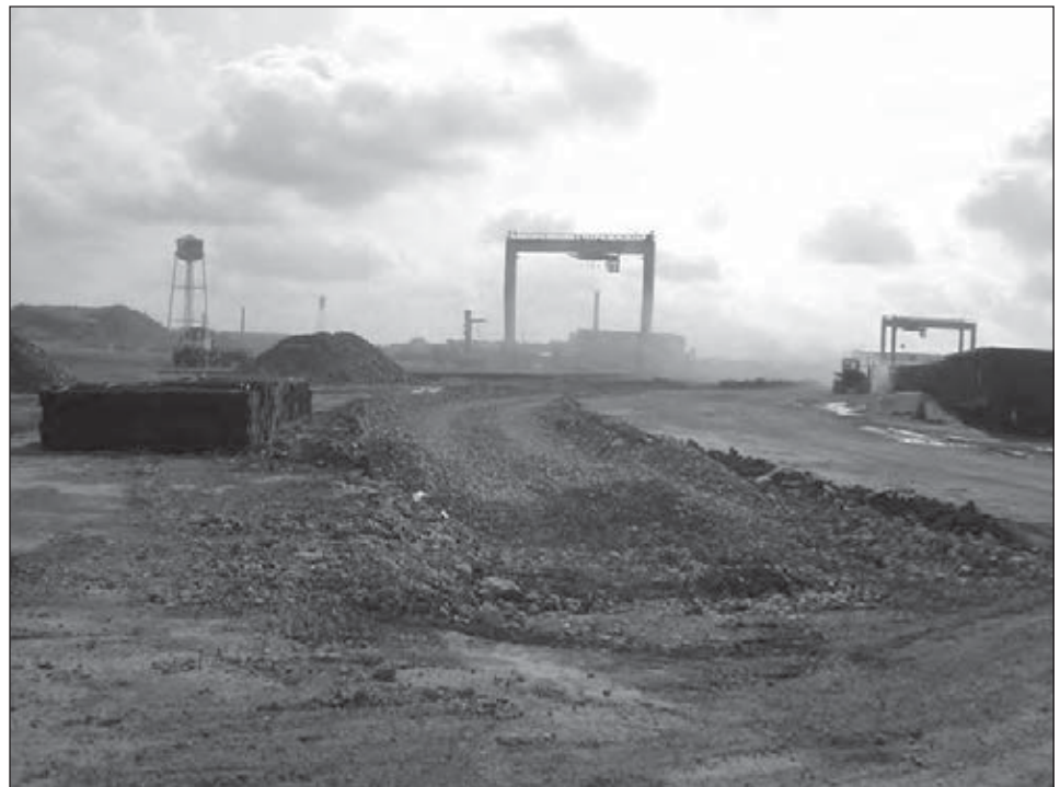
Figure 10: Digging Under Way at a Deleted Superfund Site without the EPA Site Manager s Knowledge
