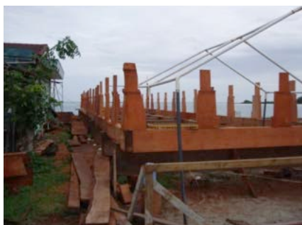
Corner post saus (on left corner) and chad posts resting on top of the longitudinal uchutem beams and the kuoku end beams.
