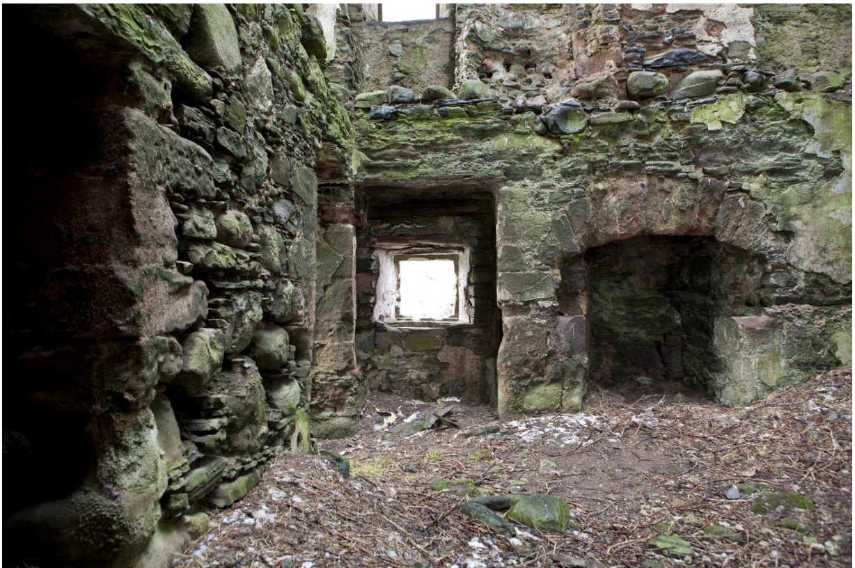
Top: the basement with its gun ports and finely constructed vault, off which the tower is built. Below: the first floor (today's kitchen).
