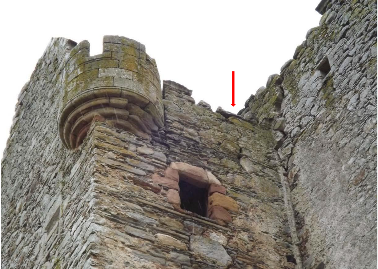
Upper parts of the early tower on the south side, showing the junction with the stair tower; location of former dormer window indicated.
