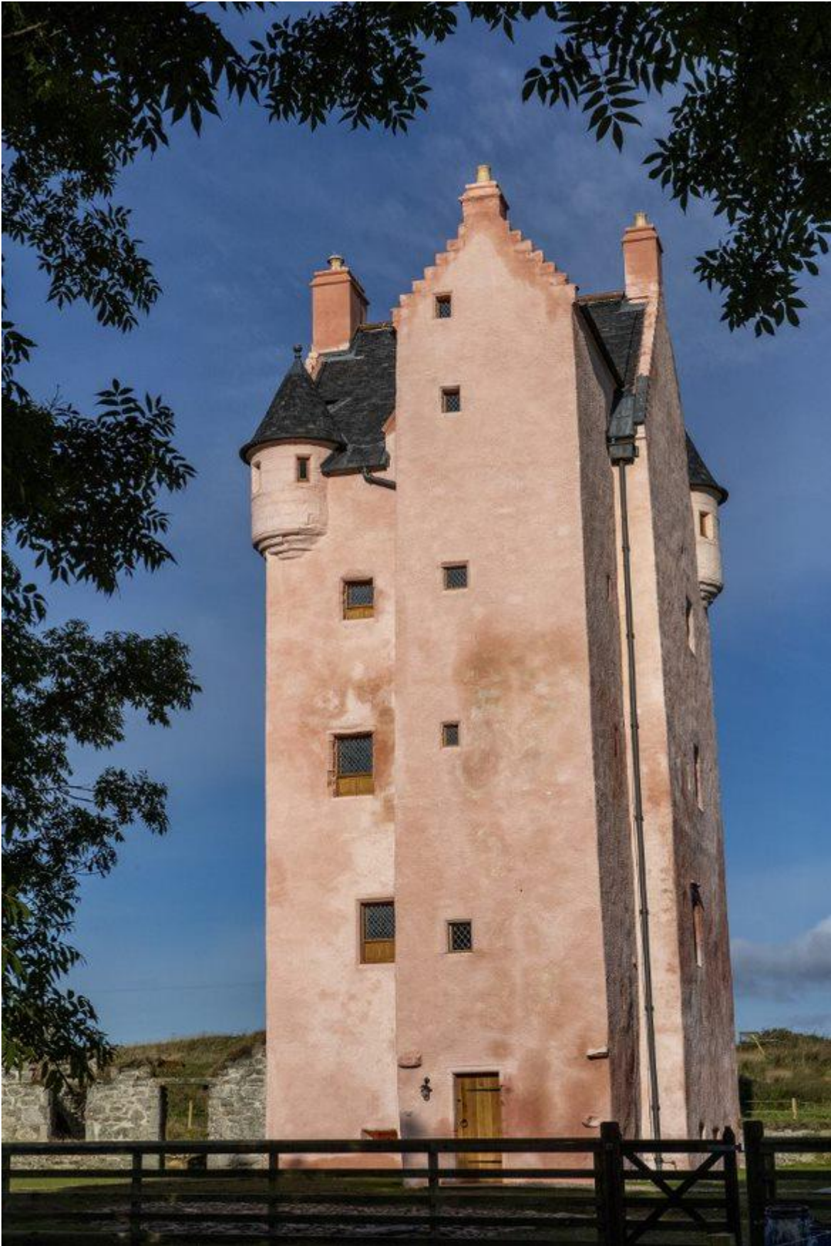
Fairburn Tower, newly completed in October 2022. (The damp patches on the exterior are caused by the differing porosity of stone beneath the render.)
