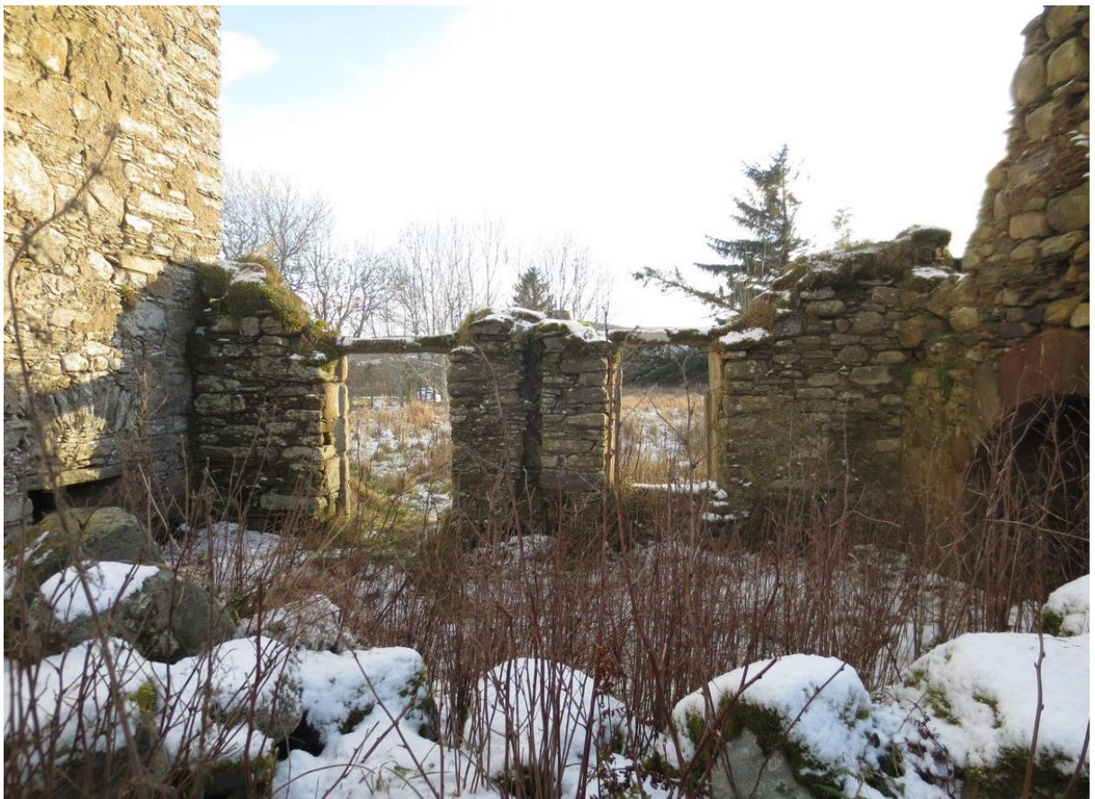
The kitchen/'dining room' range in January 2016. The position of the buried cruck frame is indicated.
