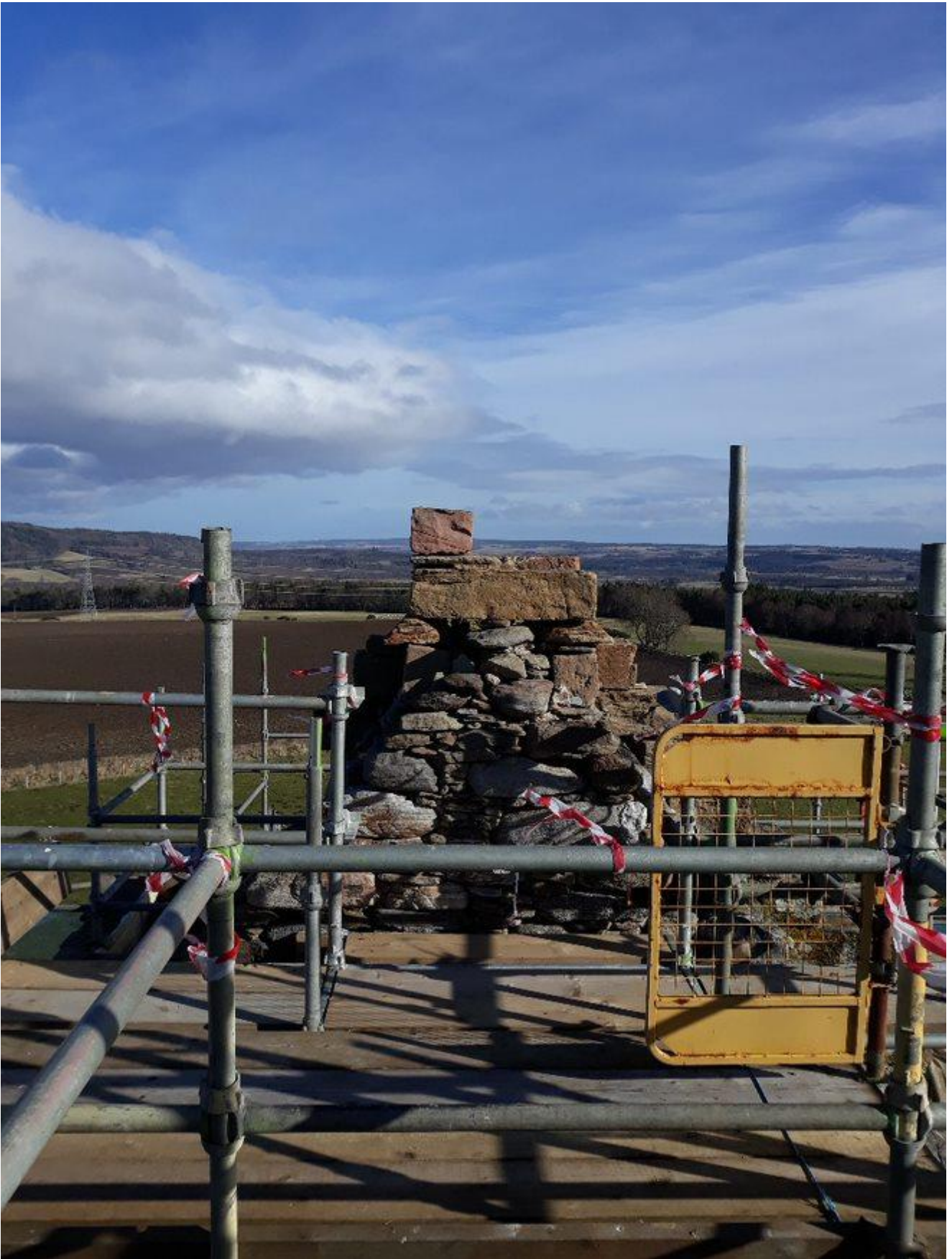
With the scaffolding in place, the views from the tower could finally be fully appreciated here at roof level.
