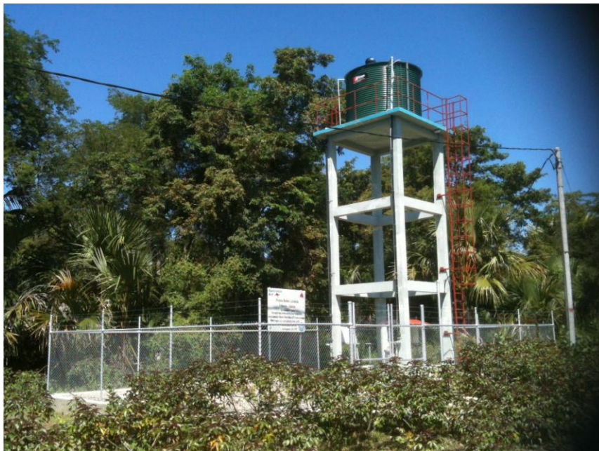
Figure 24 Caravelha Bore at Manulede River
