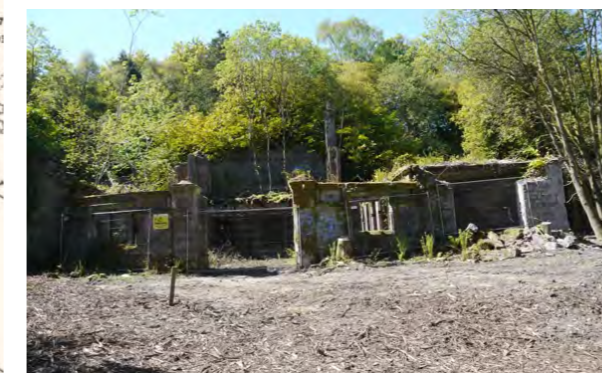
Ancillary buildings - current ruinous condition
