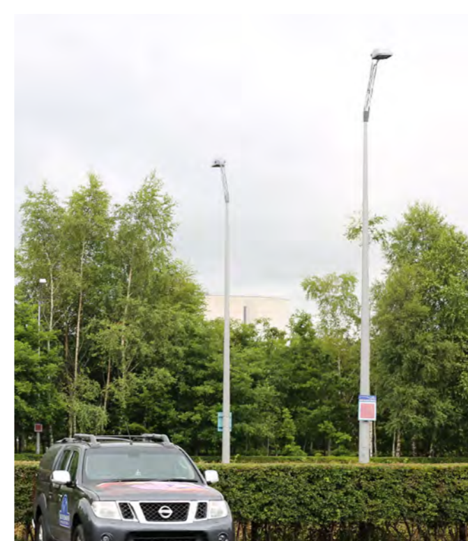
Large scale lighting columns used in car-park spaces ●
