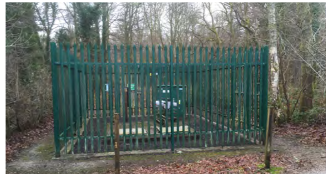
Security fencing to electrical equipment, PPC finish ●
