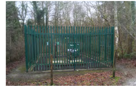
Screening of Substation required
