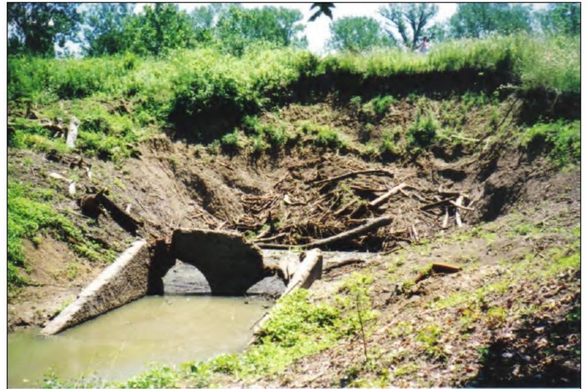
(Courtesy of USACE Louisville District) Figure 2-48. Result of successive slope failures around pipes.
