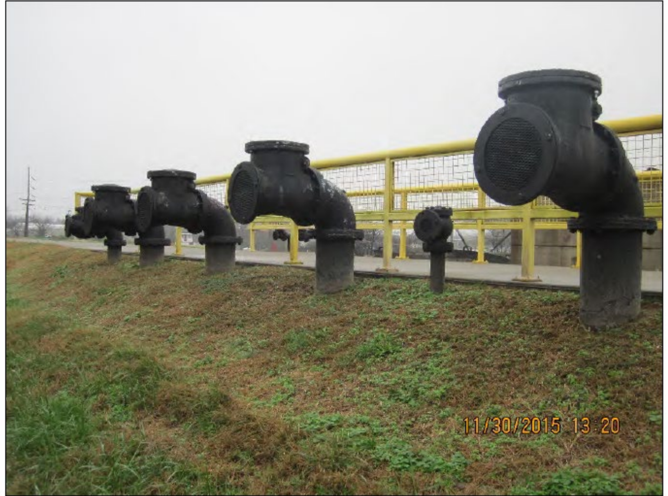
(Courtesy of USACE Louisville District) Figure 9-27. Typical pump station air vents.
