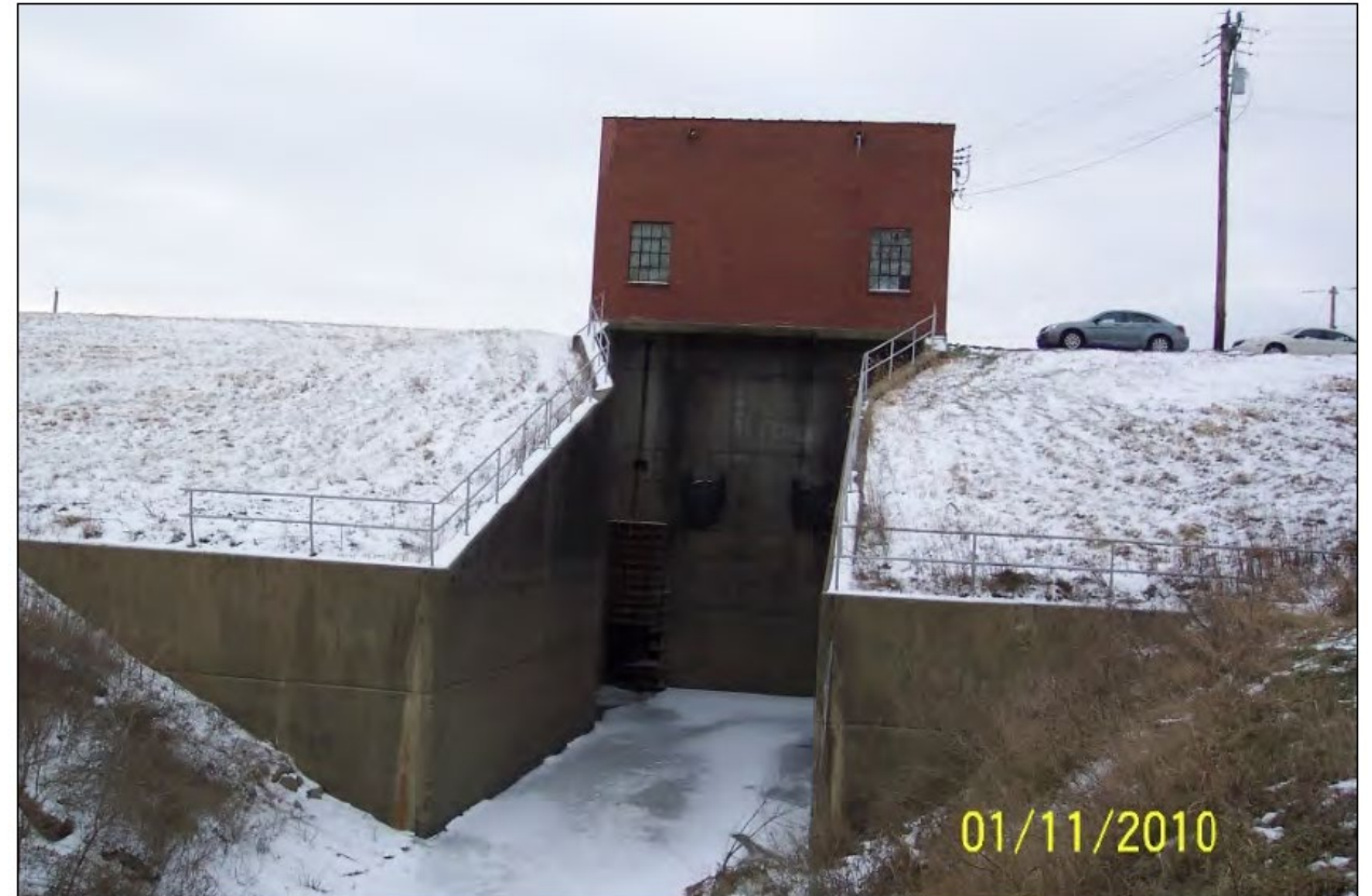
(Courtesy of USACE Louisville District) Figure 9-3. Pump station at levee centerline.
