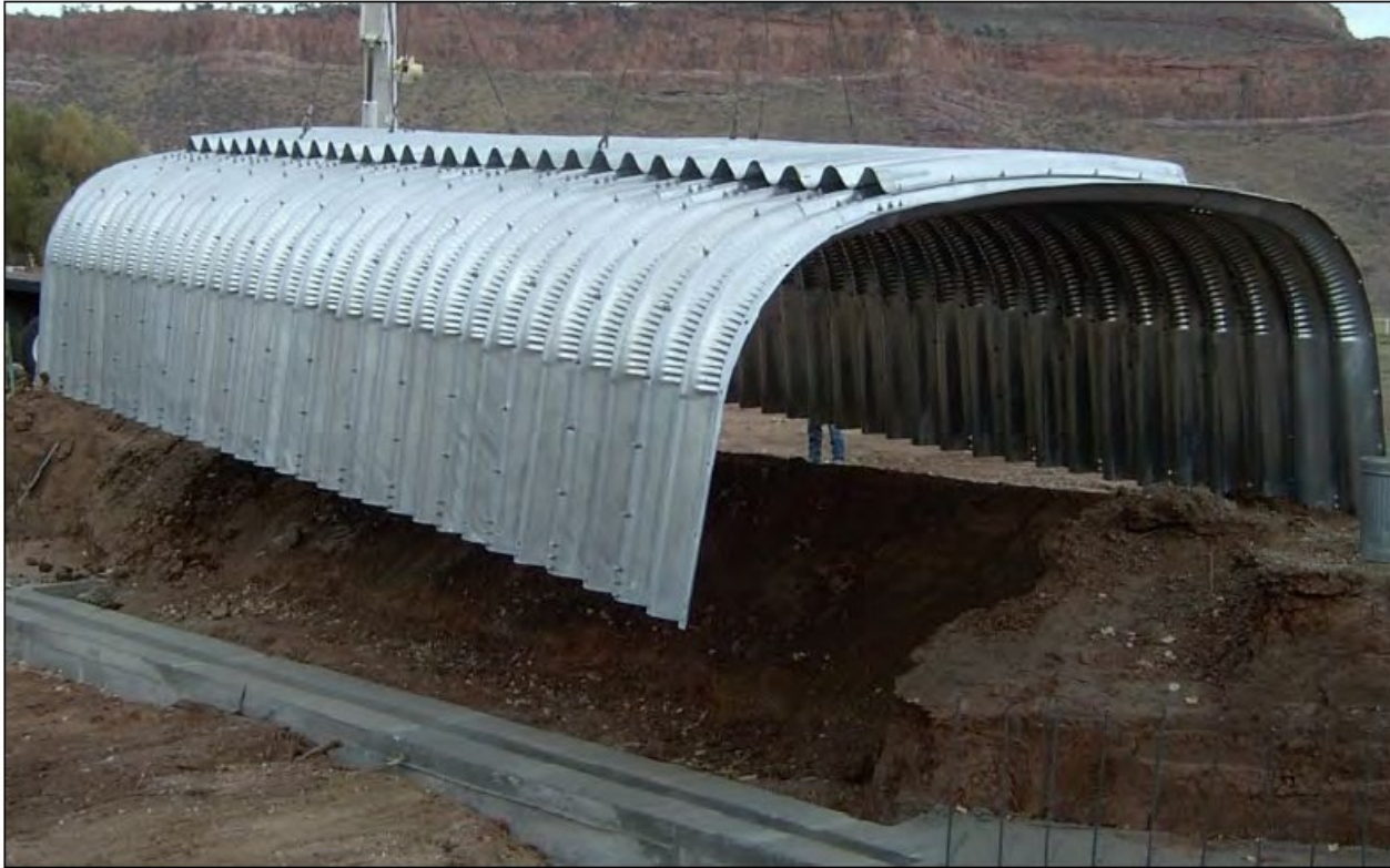
(Courtesy of National Corrugated Steel Pipe Association) Figure 3-4. Installation of a corrugated steel box culvert.
