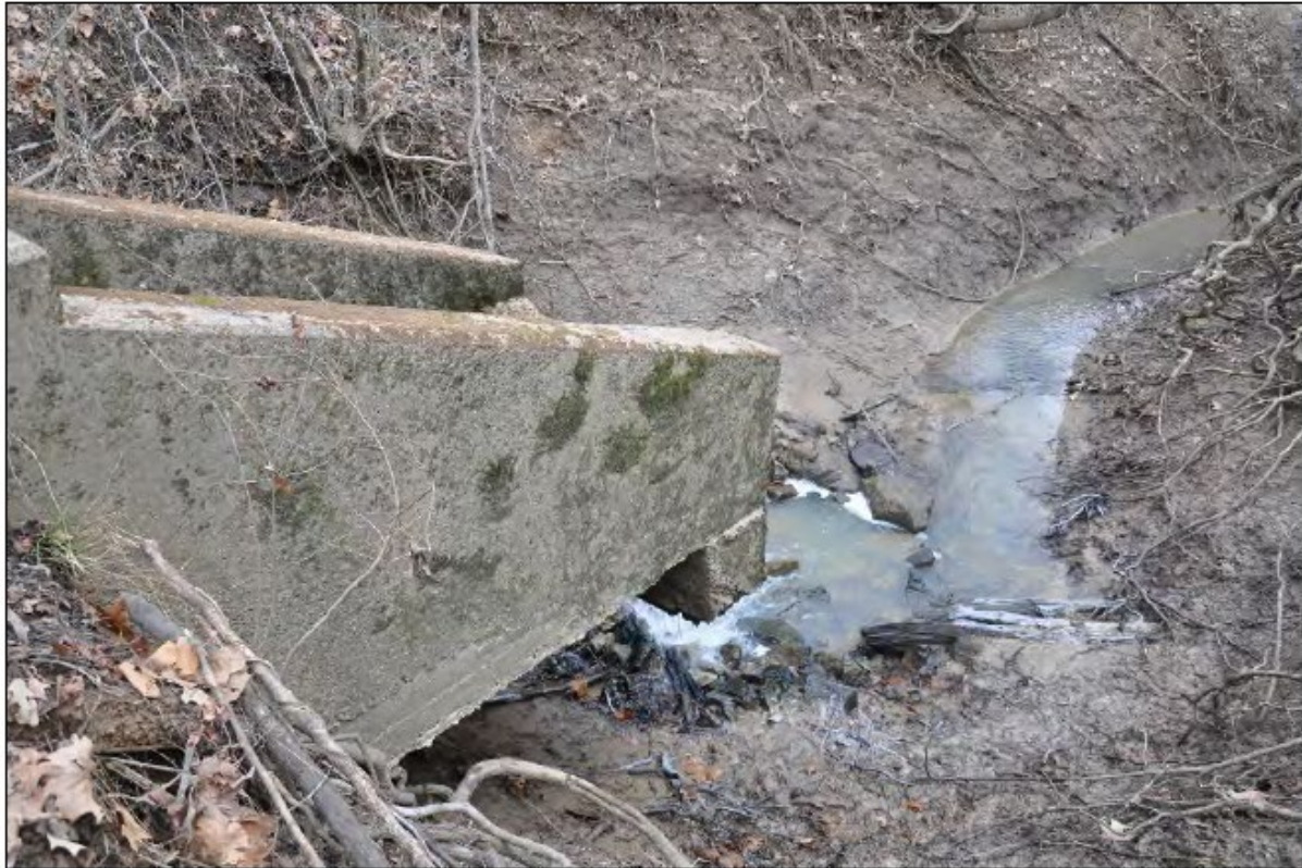
(Courtesy of USACE Louisville District) Figure 2-47. Drainage pipe outlet erosion.
