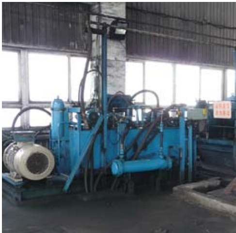
ROMJIG installation, China
