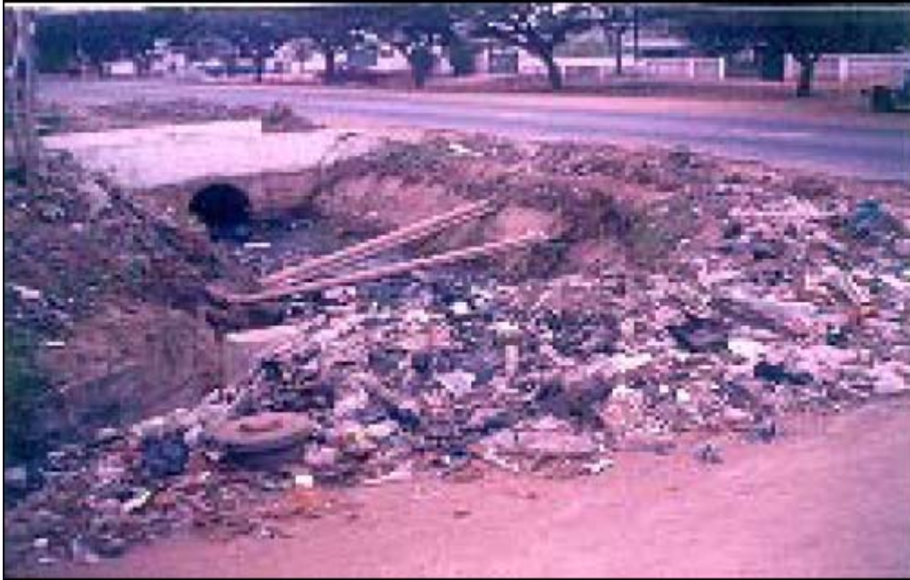
Sewage line blocked by wastes of human origin in Accra
