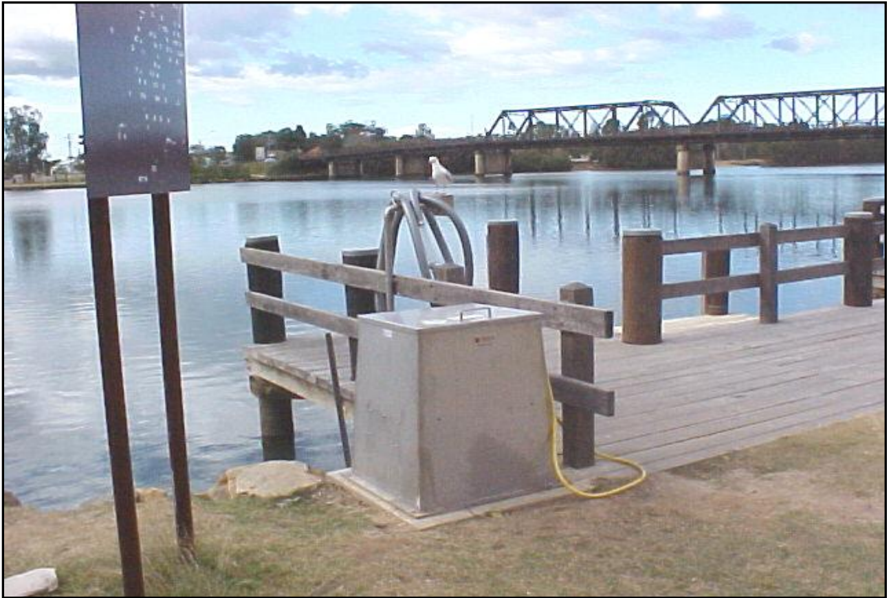
Figure 3.4: Effluent Pump-Out Station, Macksville
