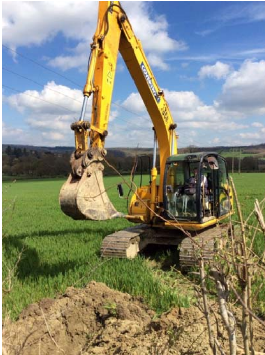
Photograph showing typical single 360 tracked excavator on site to dig out trench for pole and stay wires
