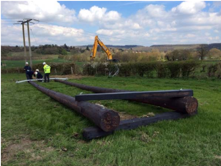
Photograph showing typical twin wood pole being prepared with reinforcing beams at pole end, to be placed underground. NB most poles used in the Proposed Development will be single.
