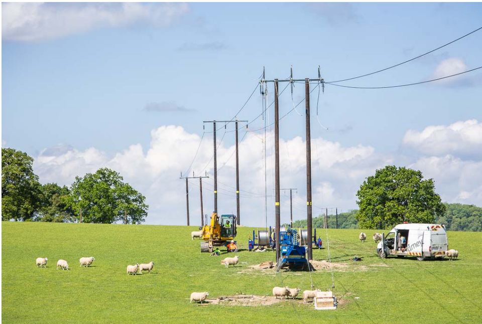
Photograph showing typical stringing activities of twin poles. NB most poles used for the Proposed Development will be single.
