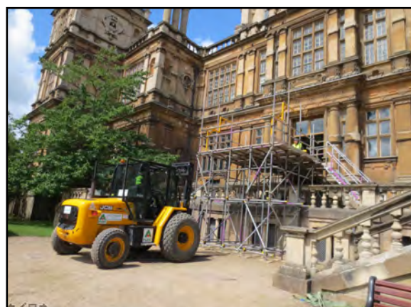
Figure 4. Scaffold platform built on the rear of Wollaton Hall during the installation (and deinstallation).
