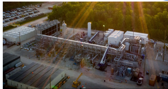
Vasu Lab helped NET Power's Allam Cycle Demo Plant
