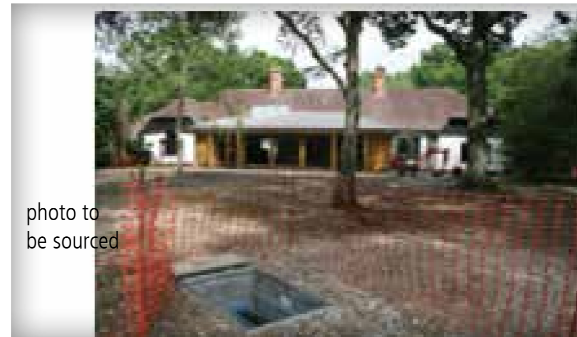
Ground source heat pump installation at Ferry Crofts Scout Activity Centre, near Beaulieu
