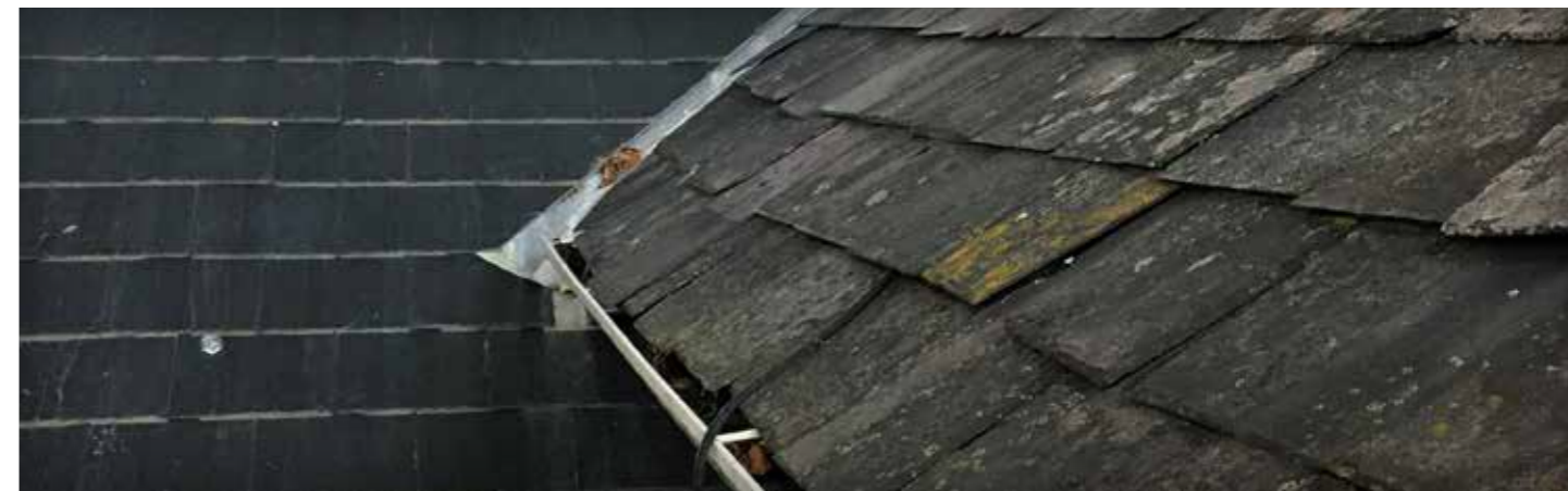
A photograph showing traditional natural slates (right) next to modern shiny slates (left)
