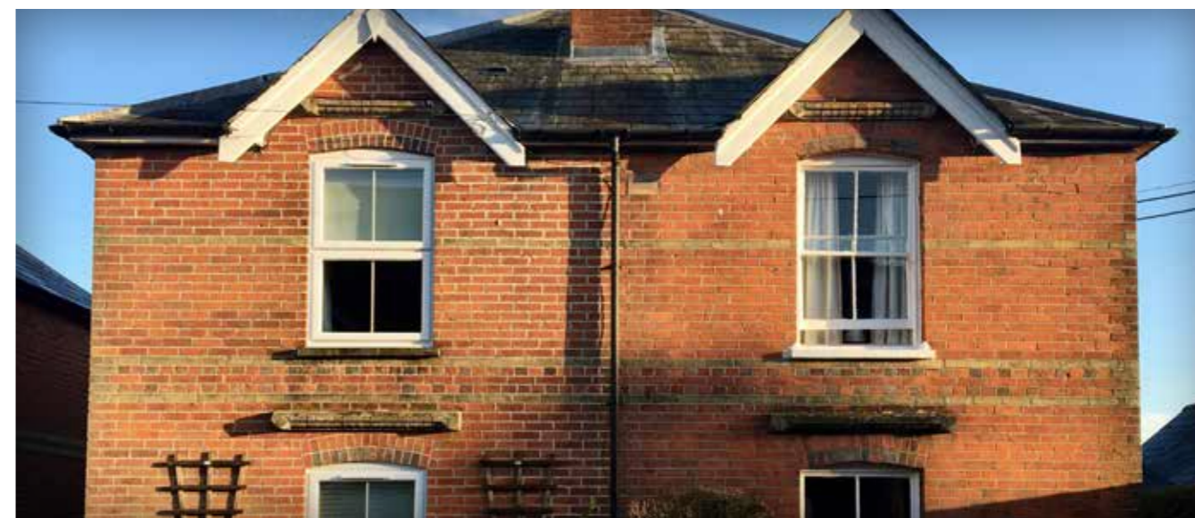
A pair of cottages showing the difference in frame size, finesse and detailing between uPVC frames and timber frames
