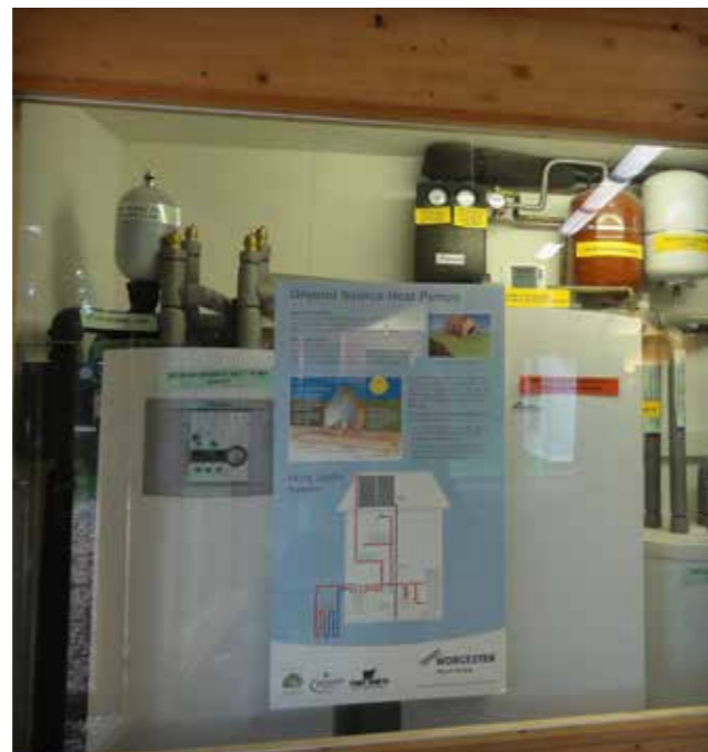
Ferry Crofts groundsource heat pump
