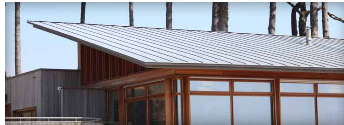
The metal standing seamed roof on the Lookout Café at Lepe Country Park
