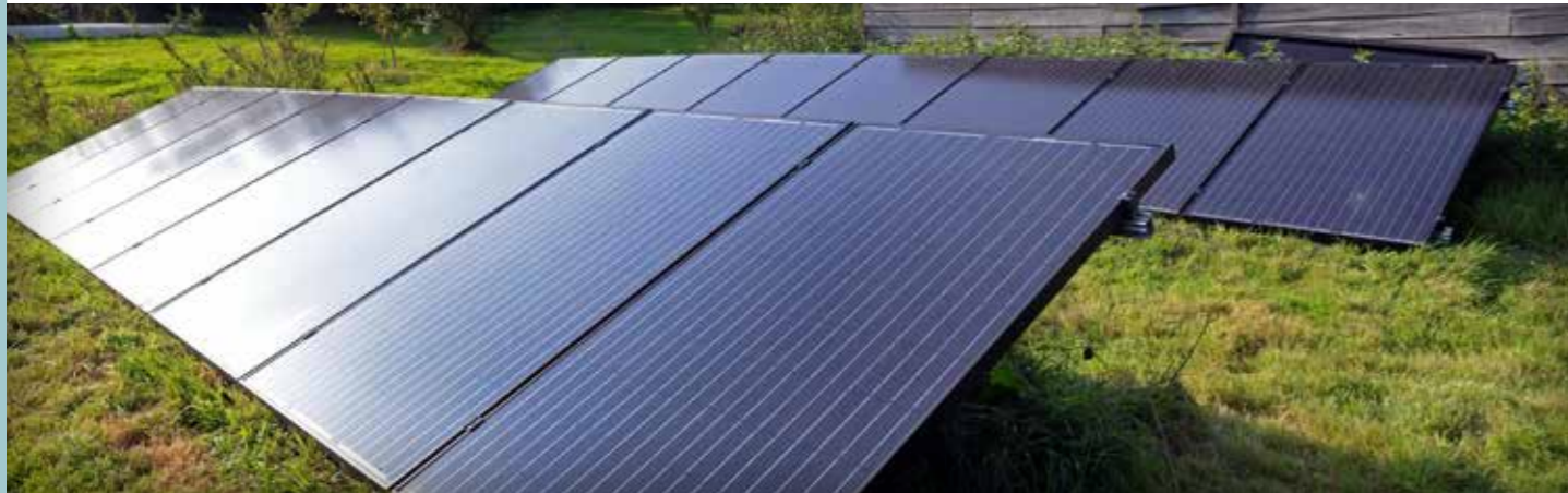
Ground mounted solar panels at Efford Mill
