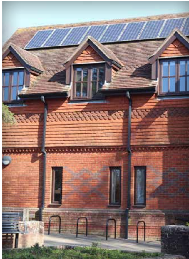
Solar panels at the New Forest Heritage Centre, Lyndhurst
