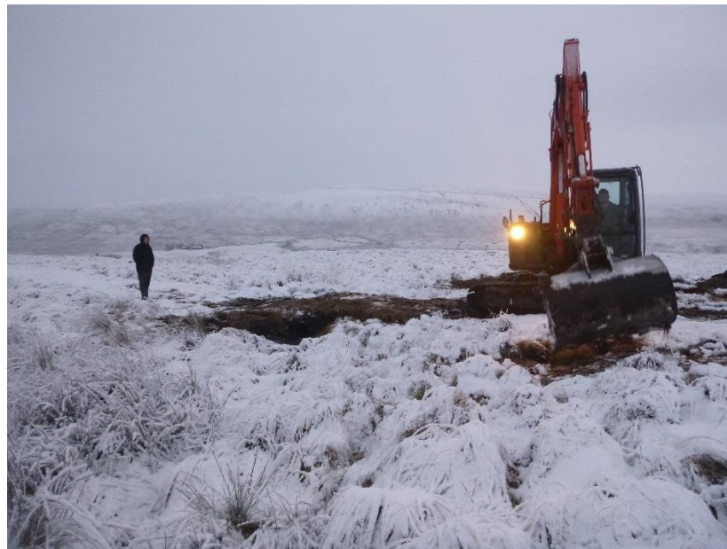
Figure 4 Contractor correcting a culverted crossing that was installed at the wrong location due to miscommunication.
