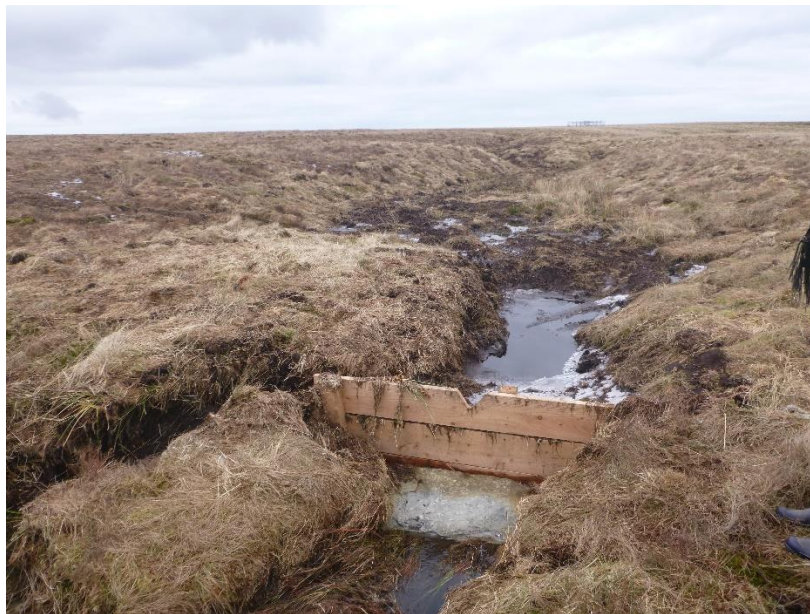
Figure 5 A wooden Sediment trap that failed not long after the contractor left site due to the design of the trap for the location. As viewed in the picture, water has eroded around the wooden sediment trap through the left bank creating a bypass channel and making the trap redundant.
