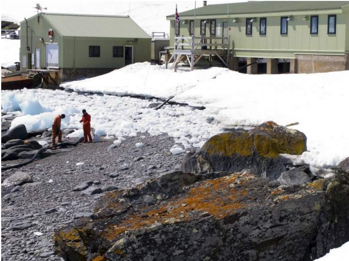
Matt and Tony attending to the loo pipe which had come loose from its anchorage aided by elephant seals and ice.
