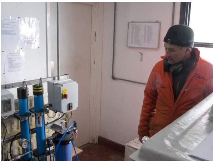
Tony Clements in the reverse osmosis shed
