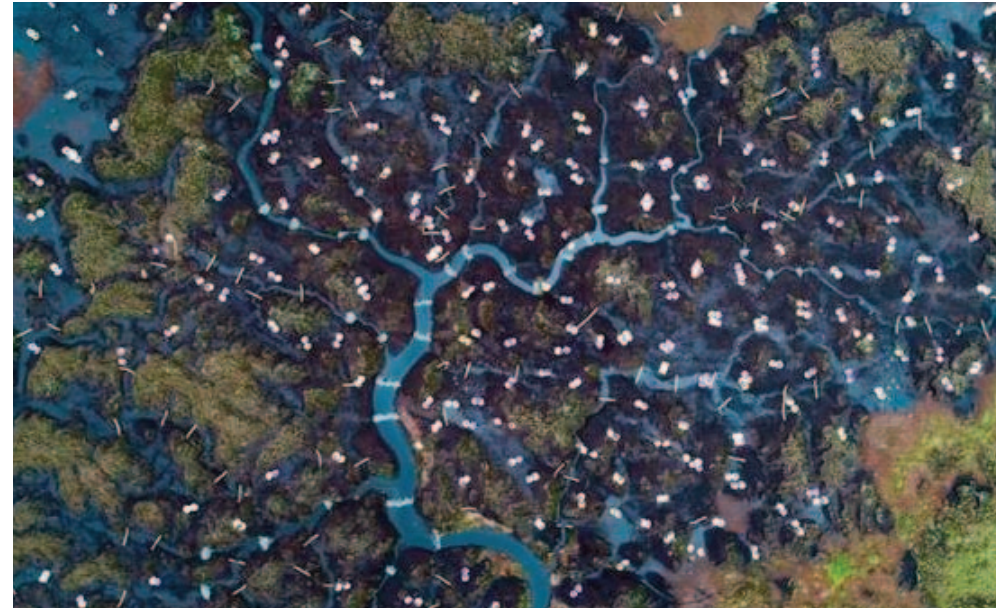
Peatland restoration in progress, showing stone dams, coir rolls and bags of brash
