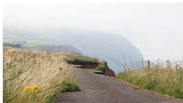
Fig.144 Coastal road lost to a landslip north of Staithes. Boulby Head is shrouded in mist in the distance.
