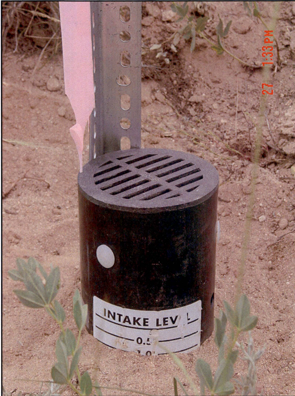
Figure 2.7-4. Stormwater sampler installed to collect a 1-L sample of snowmelt or storm surface runoff.
