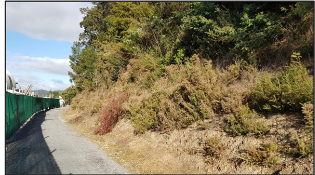
Photo 2: Vegetation on the cliff bank/landward side of cycle trail. Ashby's Boatyard on left.
