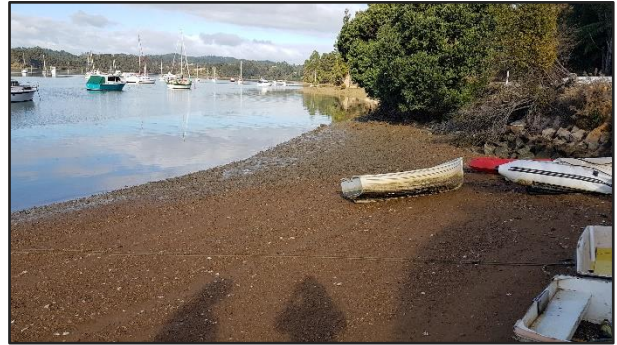
Photo 8: Intertidal area inspected, rock retaining wall which leads up to cycle trail on right.
