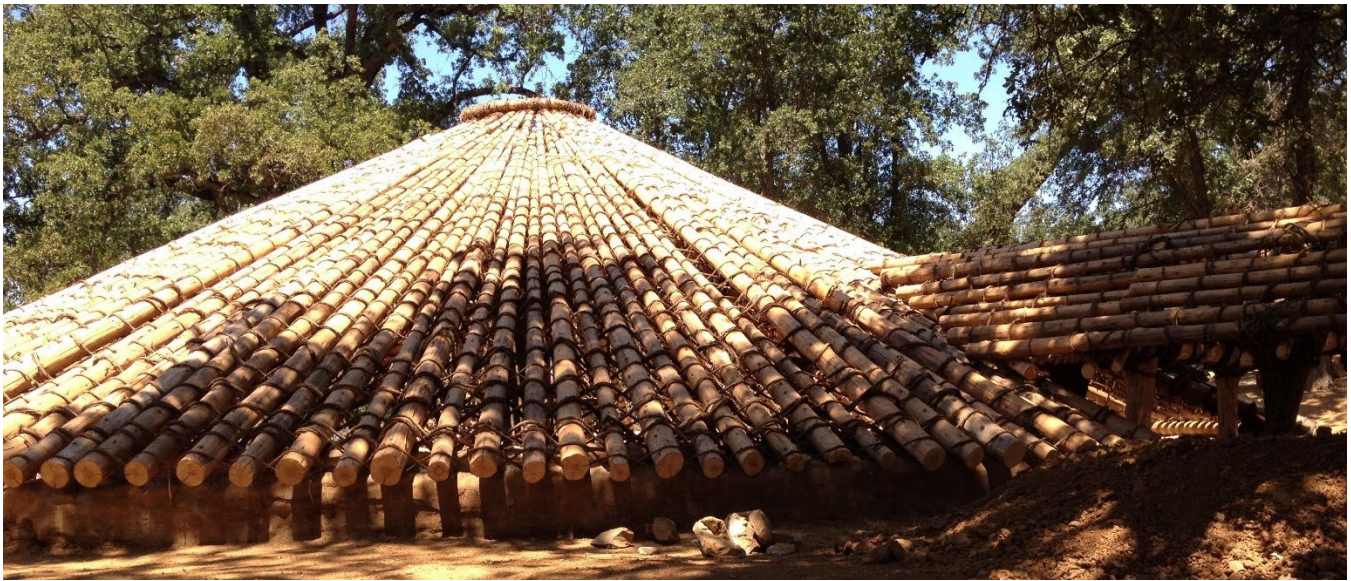
Figure 4. Miwok Ceremonial Roundhouse under construction in 2015. Note the California wild grape vines threaded through the wooden poles (incense cedar) and used to stabilize the structure. Chaw'se, Indian Grinding Rocks State Park, Volcano, CA. Photo, Margaret Smither-Kopperl.
