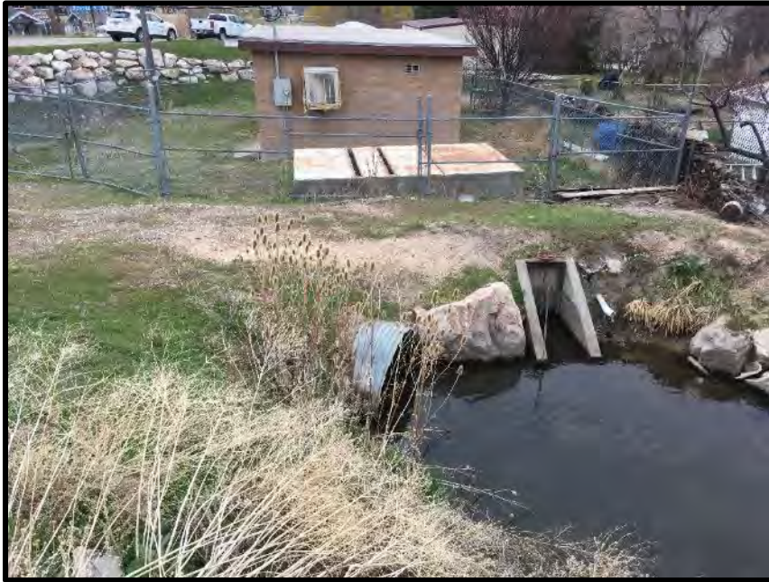
Photo 1: The beginning extent of Site 1, the North Ogden Canal existing pump station, is depicted in this photo. At this point, irrigation water enters the pipeline that would be replaced as part of the project. The pump station would be updated as well.
