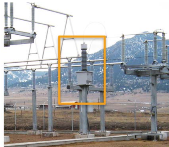
Figure 4. The 115-kV potential transformer that failed, shown here during substation construction.
