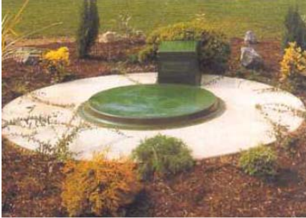
Figure 12: Installed Biocycle Unit
