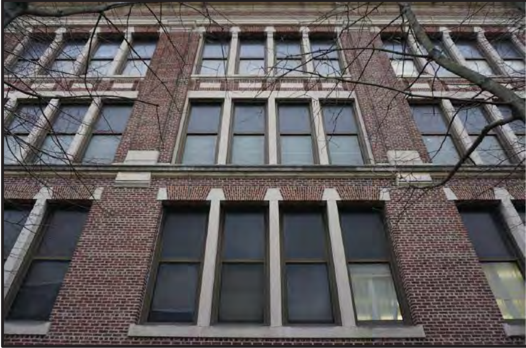
Figure 33. The southwest elevation showing the northwest end of the façade. Source: Oscar Beisert, 2018.
