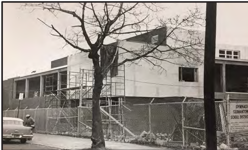
Figure 125. Looking northeast from High Street at the construction of the 1964–65 Gymnasium. Source: Photographs, Board of Education Records, CAP.
