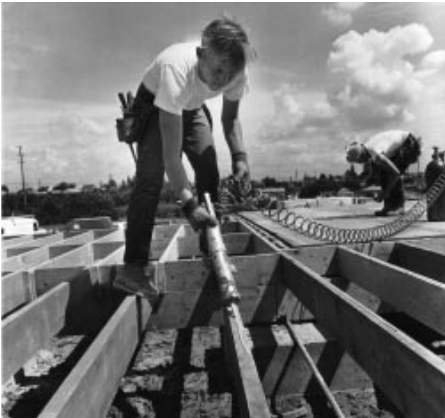
Figure 9-6. A pressurized extruder applies a single bead of elastomeric construction adhesive to floor joists for assembly of a plywood floor system.
