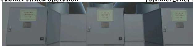
(c) Generator outlet switch and voltage transformer switching operation
