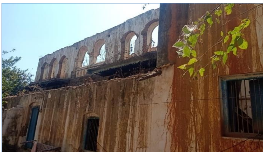
Fig. 1. The dilapidated house in Arujni-Morgaon town of Gondia district
