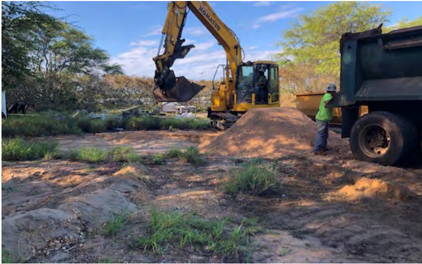
Cleanup efforts following accidental transformer oil release in 2021
