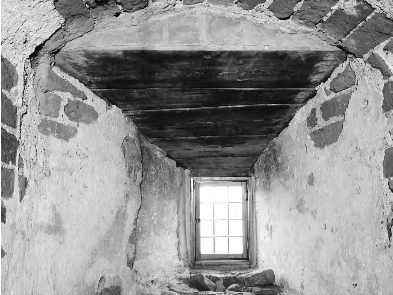
Fig. 3. Boarding of the window niche on the mezzanine floor of Häme Castle. Basing on dendrochronological analysis it is dated to the early 18th century. Photo by Terhi Mikkola / NBA, Häme Castle.
