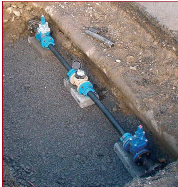
▲ Meter installation for water conservation project
