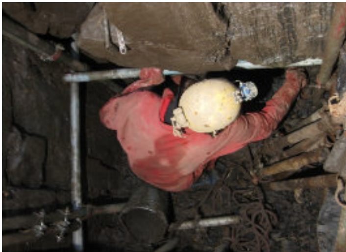
Ben Stevens installs a scaffold cage in the Tripod Dig (©Tony Baker)
