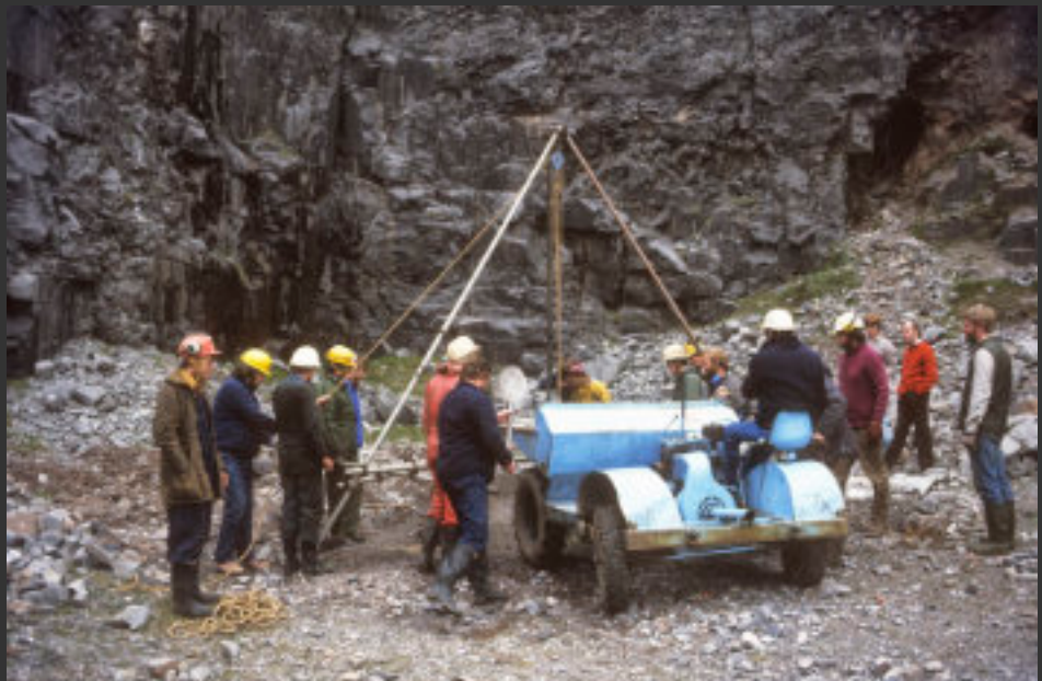
The dumper truck was a valuable tool. It was employed to shift spoil well away from the worksite
