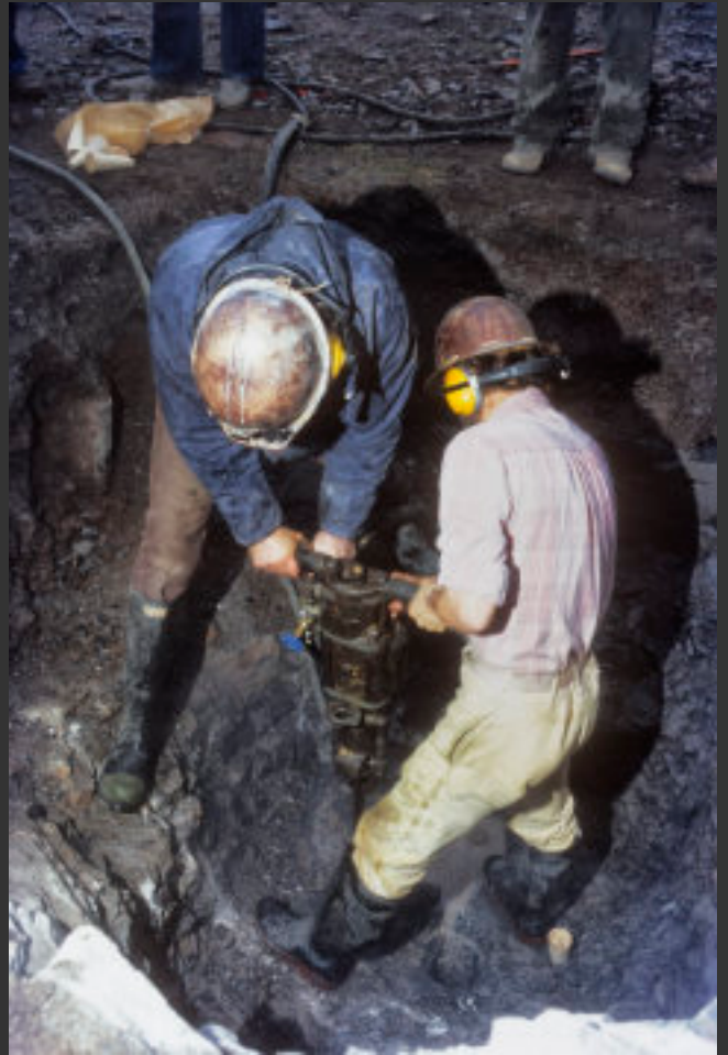
The night shift in action. The borehole clearly visible between John's feet
