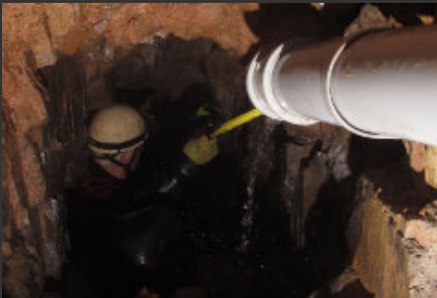
Above: Paul Quill measures up for his clever pipework, that keeps the digger dry at the sharp end.
