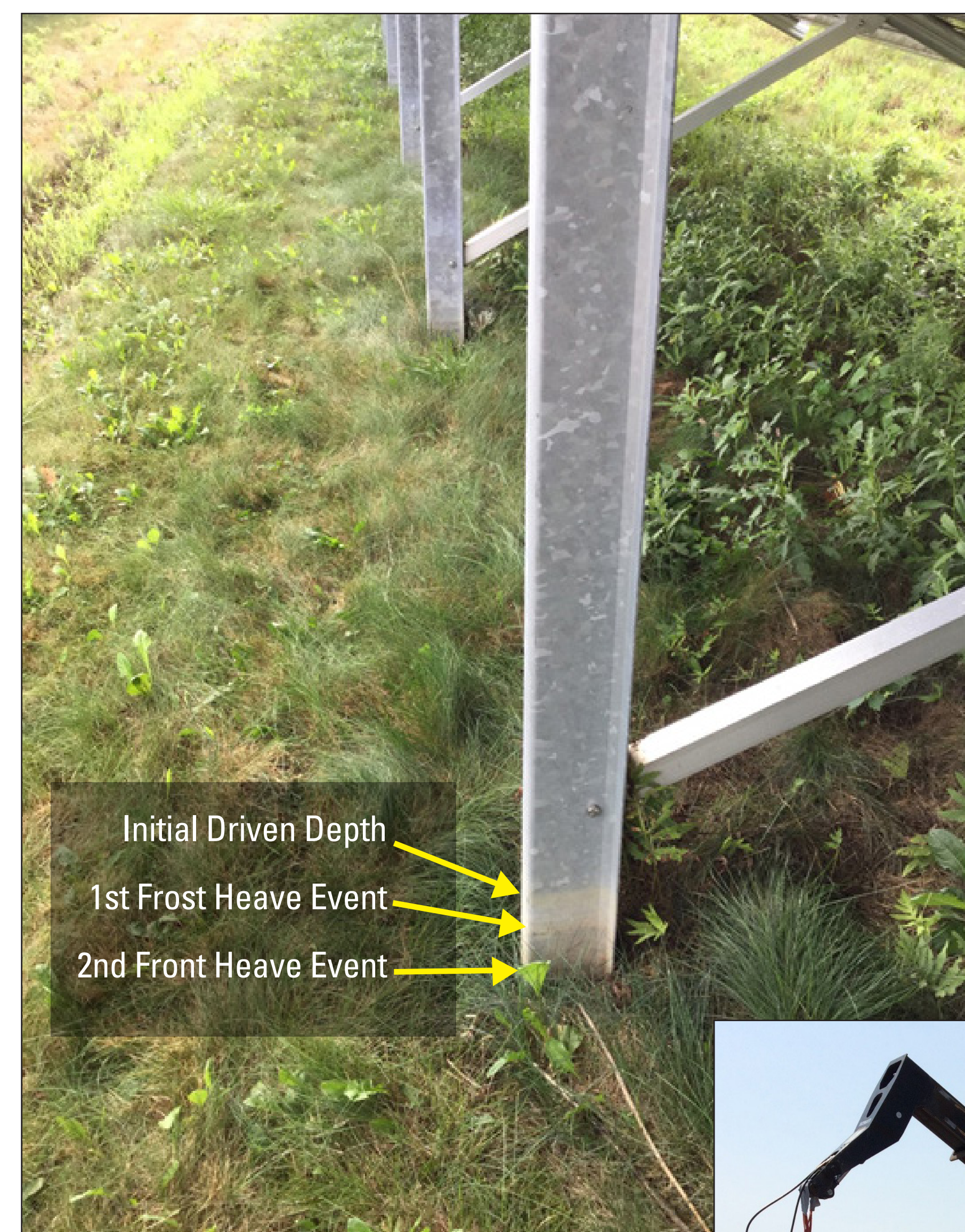
◀ Example of pile having been uplifted due to frost heave. This pile is slowly being "ice jacked" out of the ground.
