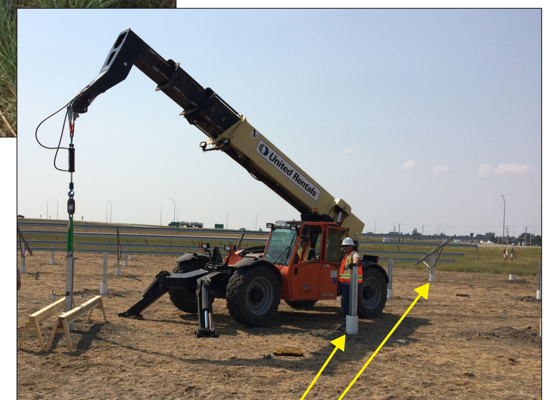
▲ PVC sleeve filled with pea gravel. PVC with pea gravel isolation of pile from adfreeze soil in frost zone.
