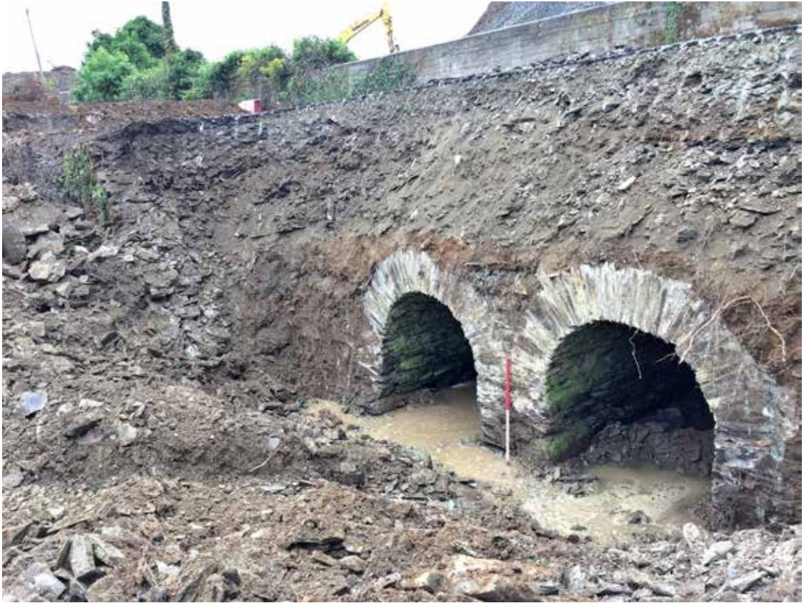
Illus. 8.6 Ballymacar Bridge phase 1 downstream elevation revealed during demolition; the phase 2 causeway revetment wall is visible in section to the left of the bridge arches (IAC Ltd).
