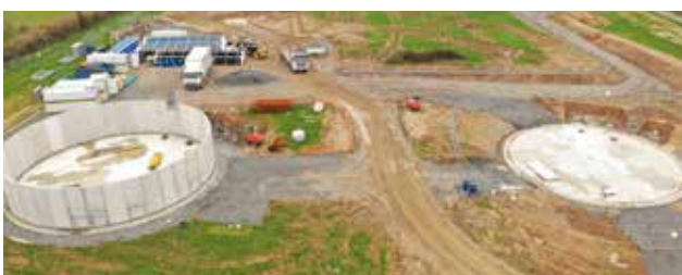
Thurles Regional Water Supply Scheme -Water Treatment Plant under construction at Bohernacrusha, Holycross, Thurles
