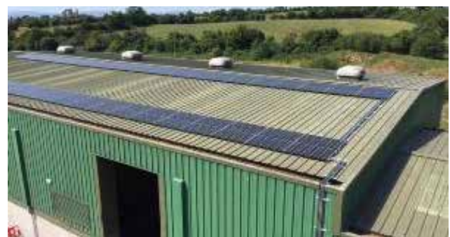
Solar Panels – Wallers Lot CAS Cashel
