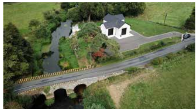
Thurles Regional Water Supply Scheme Water Scheme - Intake completed at Rathkennan, Holycross, Thurles
