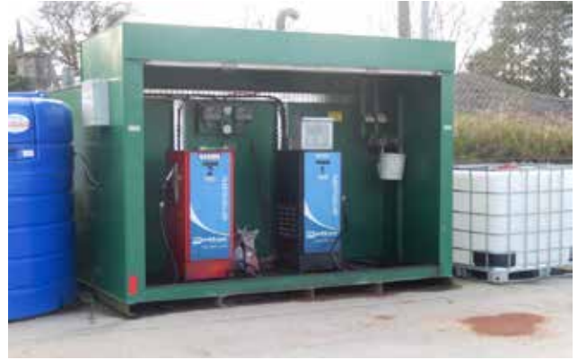
Self contained and banded fuel storage tanks and dispensing system
