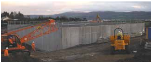
Clonmel Town and Rural Water Supply Scheme - Reservoir at Giantsgrave, Clonmel under construction
