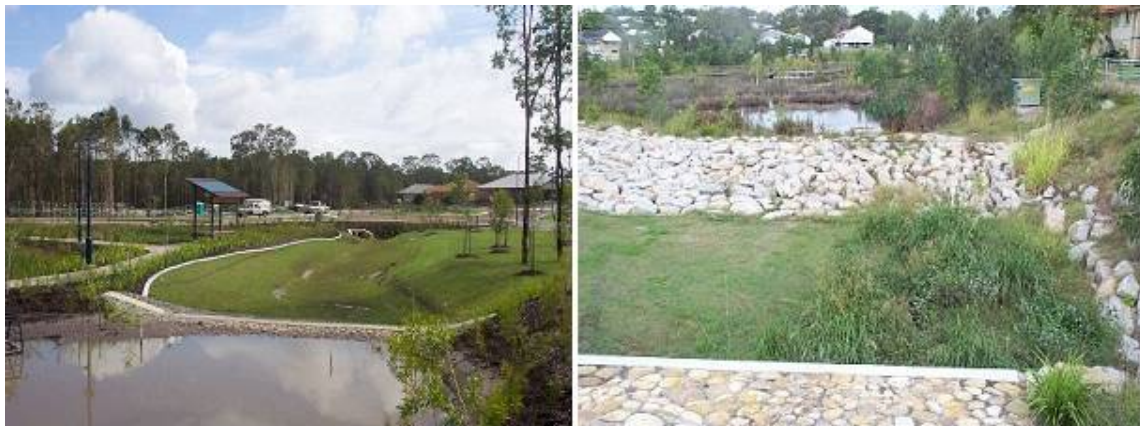
Plate 4-4: Spillway outlet weir structure of sedimentation basins at the Gold Coast and Coorparoo
