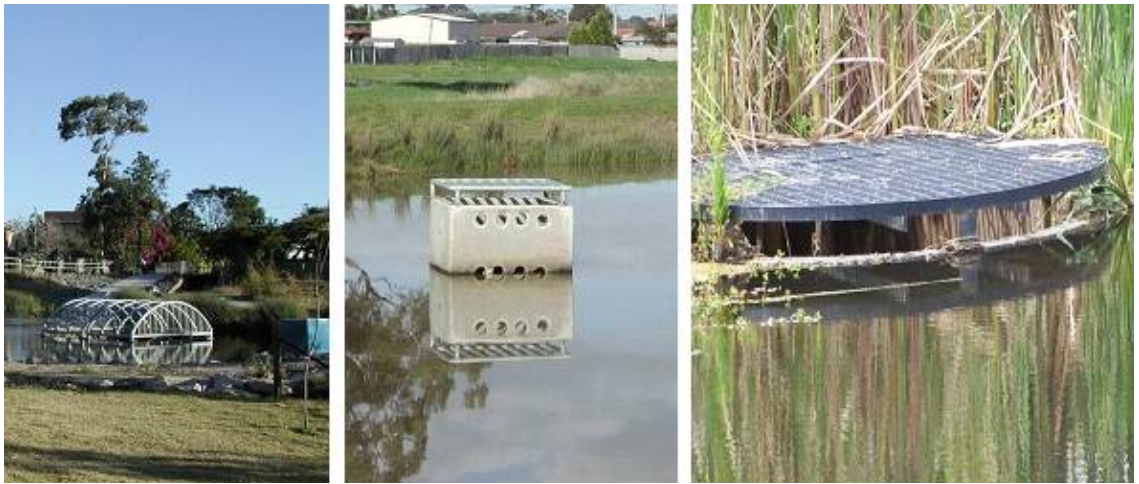
Plate 4-3: Debris screens in Coorparoo, Mill Park (Victoria) and Herston
