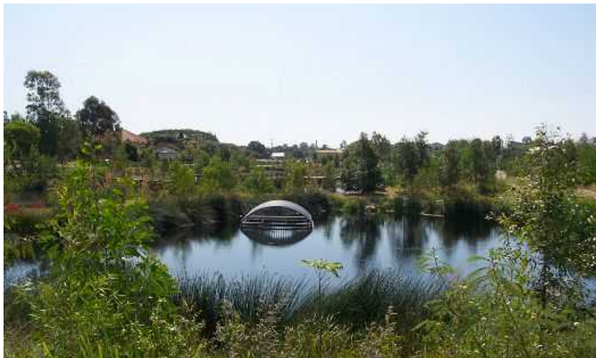
Figure 4-8: Example layout (top) of sedimentation basin 'control' overflow pit and pipe connection to a macrophyte zone and control overflow pit installation (bottom)
