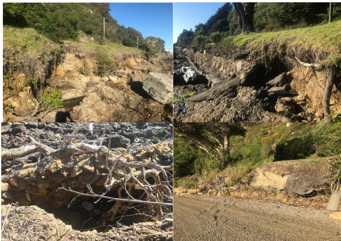
Figure 4-3: Erosion trends along the coastal line of Shelly Bay Road
