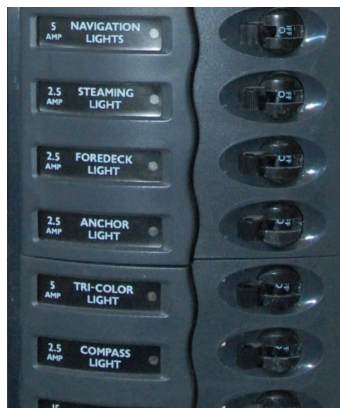
Figure 6-1 DC Distribution Panel - Center Column
