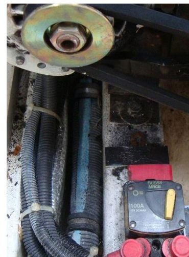
Figure 4-12 100-amp Alternator Breaker
