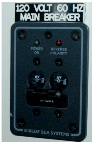
Fig 1-19 AC Main Breaker Panel - Aft Compartment
