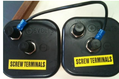
Figure 4-19 6V Batteries in Series
