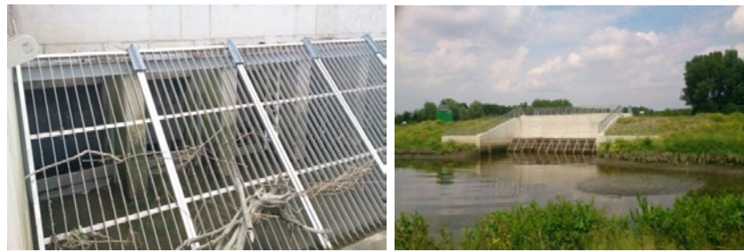
Figure 6 View of the inlet sluices from the river side (on the left) and inlet and outlet sluices from the FCA side (on the right)
