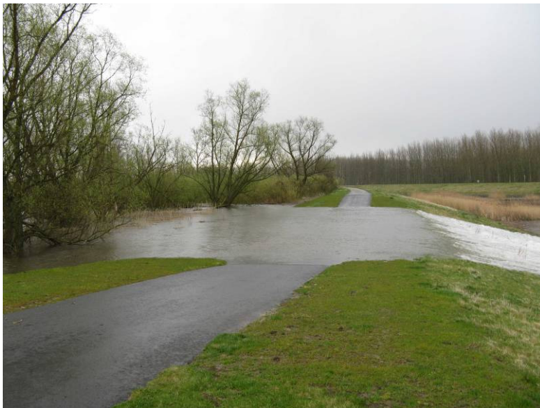
Photo 1. Lowered overflow dike of Lippenbroek in action.
