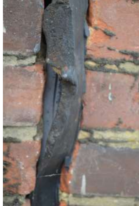
Figure 6.19: Join between the two buildings, showing a rubberised infill and also polystyrene behind.
