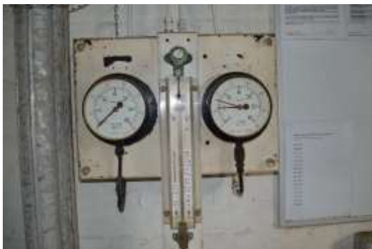
Figure 6.29: Original valve board on party wall between the Northern and Southern Buildings.
