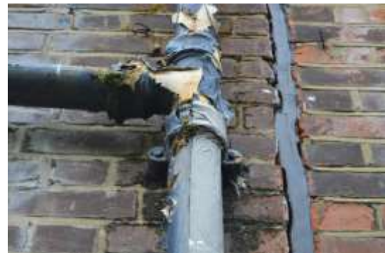
Figure 6.15: Note the junction between the two buildings. The brickwork between the two buildings is not bonded together.
