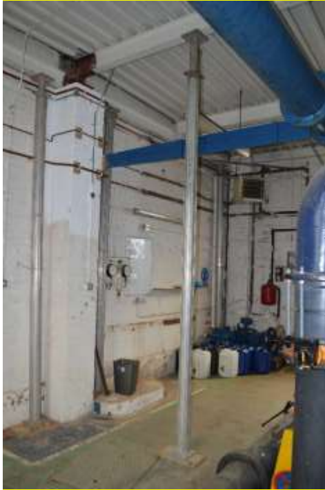
Figure 6.21: The building's roof shows signs of substantial structural problems and is currently propped in a number of places using temporary Acrow props.
