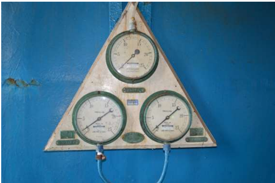
Figure 6.13: Original Royles valve board to the original Royles cylinders.
