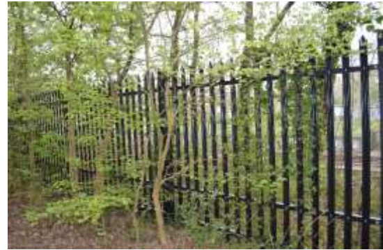
Figure 6.7: View of the metal fence along the most westerly footpath within the woodland, adjoining the railway track. Note very limited visibility through westwards to the Site.
