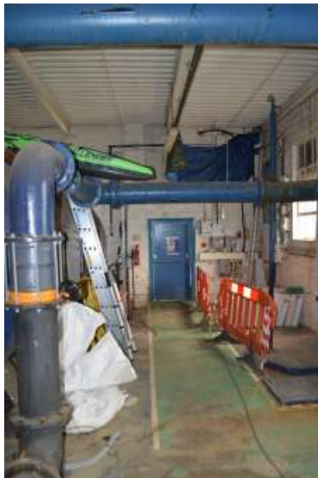
Figure 6.23: Main corridor, leading to the southern elevation. Shows the main water pipe to the cylinders.
