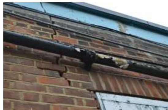
Figure 6.17: An example of a significant structural crack to the eastern elevation.
