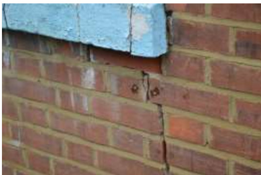
Figure 6.16: Significant structural cracks in many areas across the elevation and residual evidence of the use of Avonguard crack monitoring equipment.
